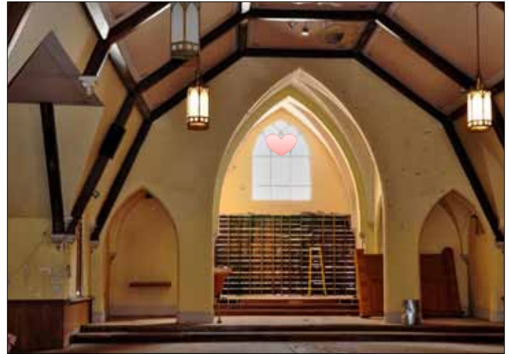
The former sanctuary, above, will house the majority of the library and will be finished with money raised by the Friends of the South Berwick Library.
