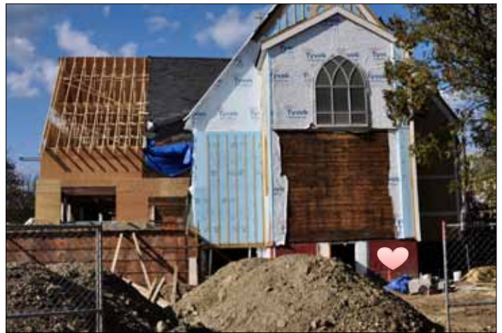
Dave Stansfield (top) and renovations to the former St. Michael's Church, soon to be the new site of the new South Berwick Library.
